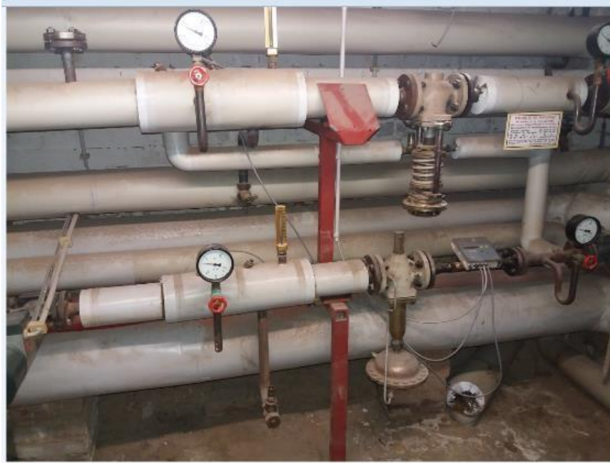
Figure 128: District heating transfer station
