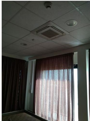
Figure 15: 4-Way Cassette indoor unit placed in Smart House Building
